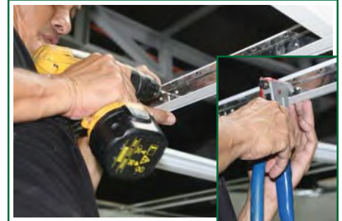
Step 3 - From the outside drill & rivet the Conversion Box Frame to the upright of the ceiling grid on 2 opposite sides.
